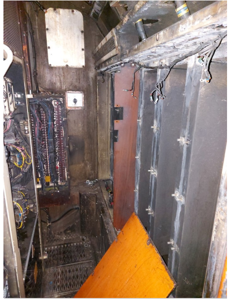
Above: A typical scene inside the power car showing missing main rectifier, but as with the other parts a complete rectifier was provided by EMR, which later in the week had turned into the scene below
